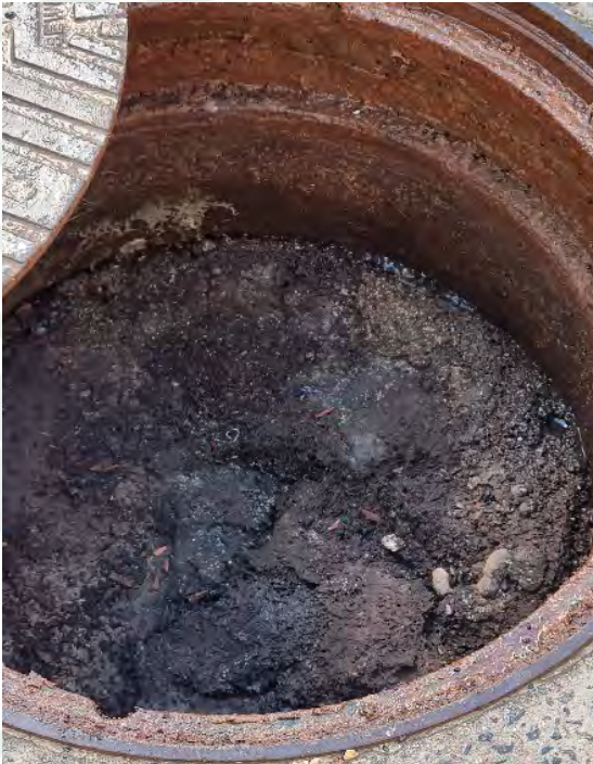
No GA, ST blocked by grease
