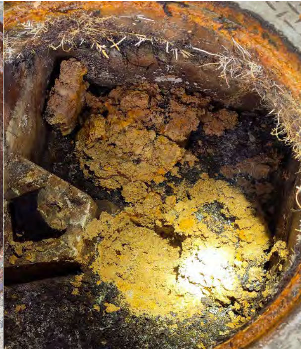
GA blocked by grease
