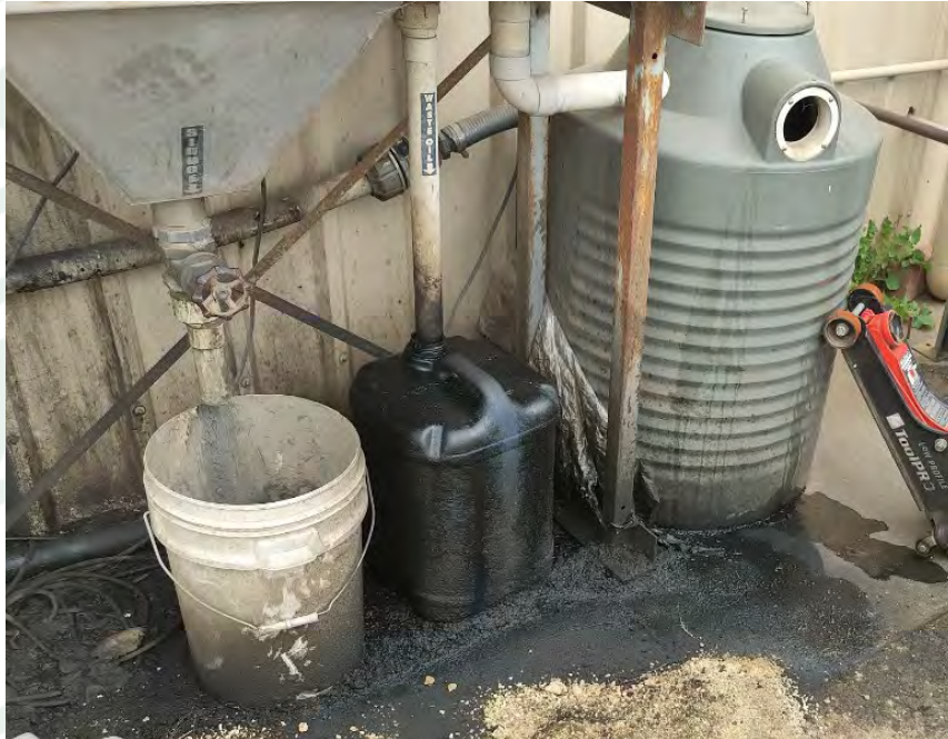
Poorly maintained oil water separator
