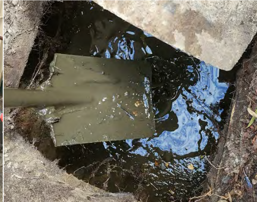
Septic tank full of oil
