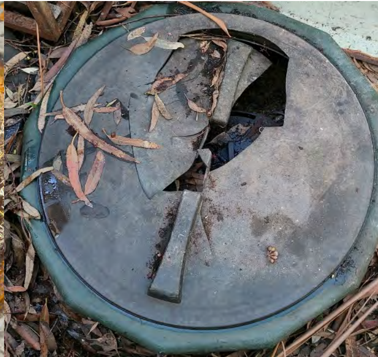
Damaged and undersized
